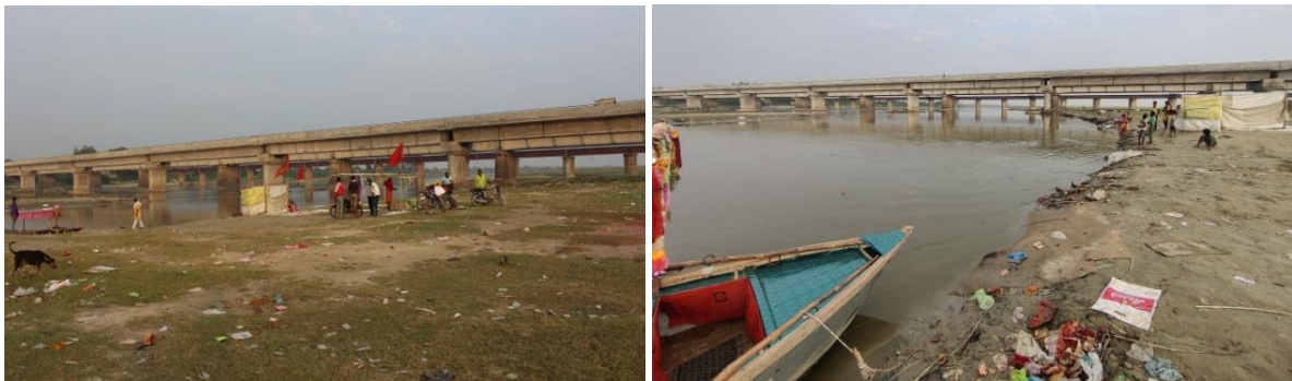
Figure 5-1: Dilapidated Ghat along river edge and connecting bridge (left), Vacant Land Parcel near bridge (right)
